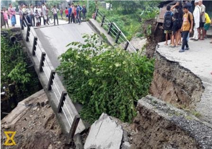
Bridge at Dhankute road in Dharan collapses Sep 25, 2015 (Kantipur News)
