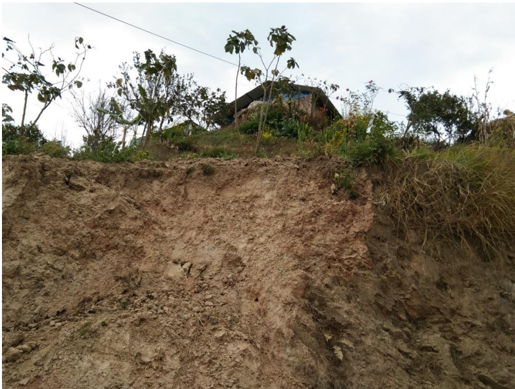
Photo 6: Road construction-induced soil erosion in Kavrebhanjyang.
