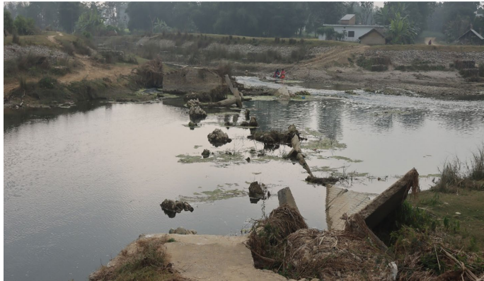
Photo 50: Destruction of physical infrastructures caused by flood of Dolai River
