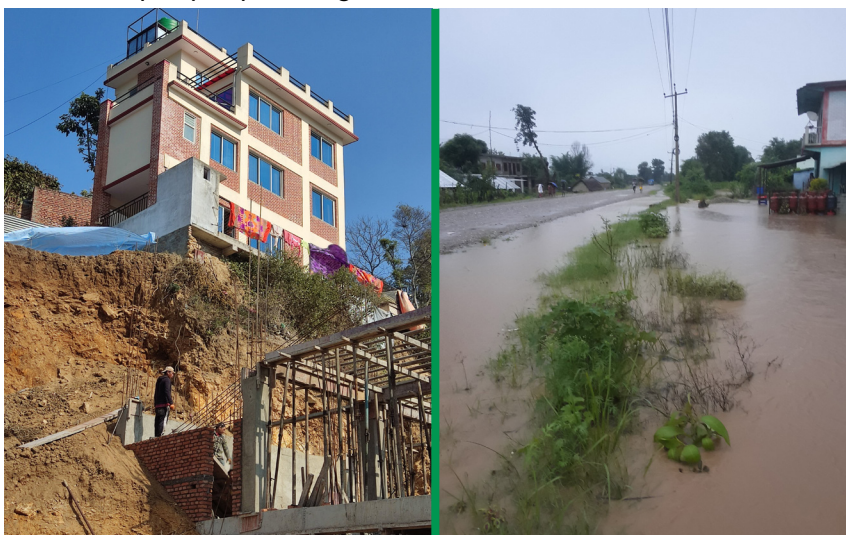
Photos: The haphazard construction risking both upper and lower buildings in Khokana (left) and the poor drainage alongside the road leading to inundation of settlements in Rapti (right)
